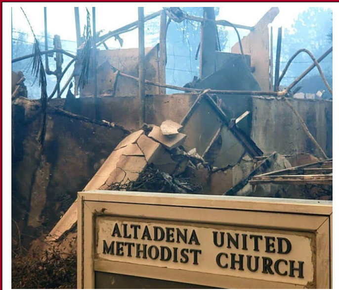
The sign still stands for Altadena United Methodist Church in Altadena, Calif., but not much else after wildfires devastated the area. Photo by the Rev. Garth Gilliam, district superintendent, California-Pacific Conference
